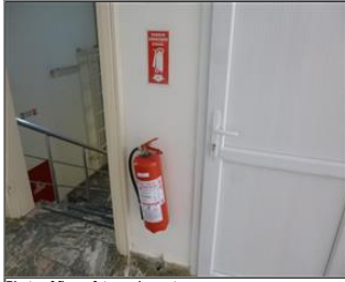
Photo of fire safety equipment Fire extinguisher.JPG
