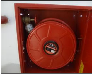
Photo of fire safety equipment Fire hose.JPG
